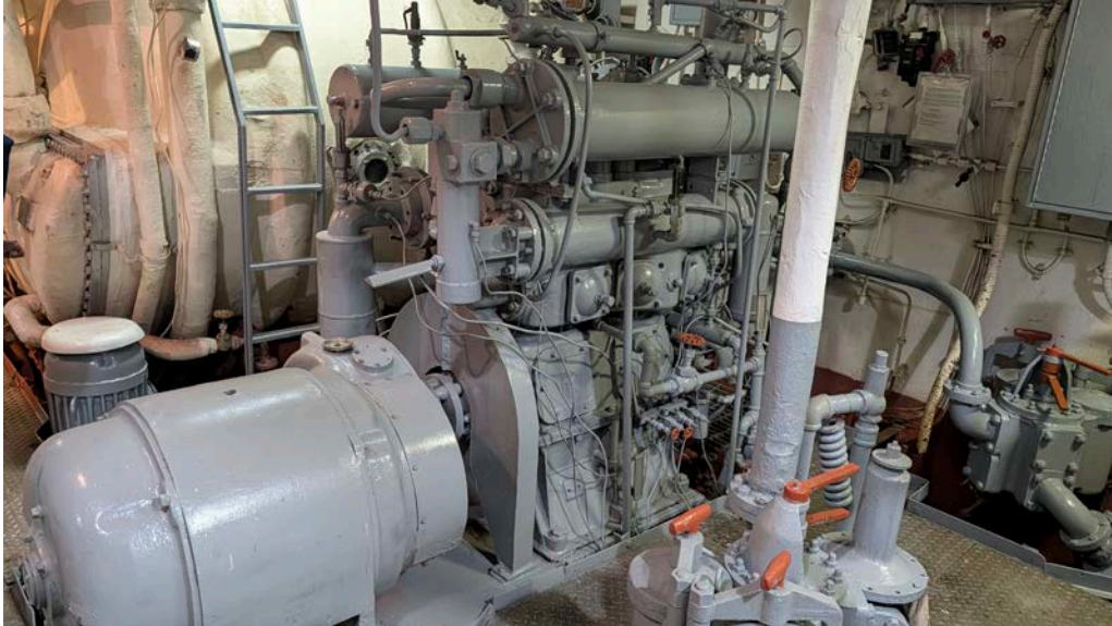
Figure 13 300 PSI Air Compressors
