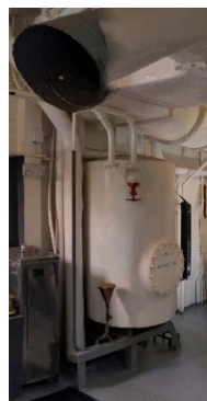
Figure 3 Lube Oil Storage Tank
