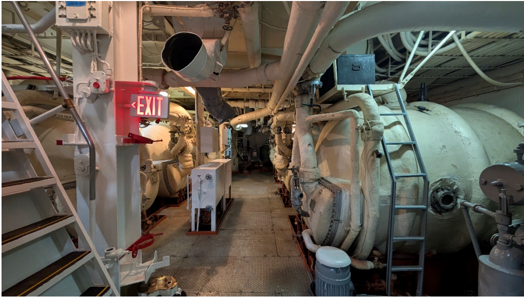
Figure 10 6th Deck Evaporator Row
