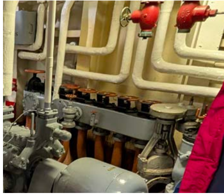
Figure 6 Bunker C Manifolds
